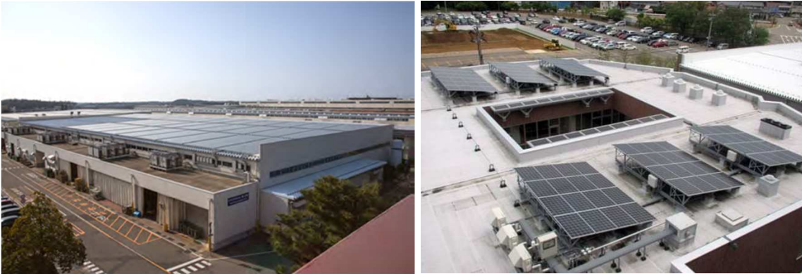
Picture-4 Project B-2)( i ) Solar PVs (example, Awazu Plant, Roof top type)
