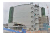
One of Japan's Largest LNG Tanks under Construction (At the Ehime Works Site)
