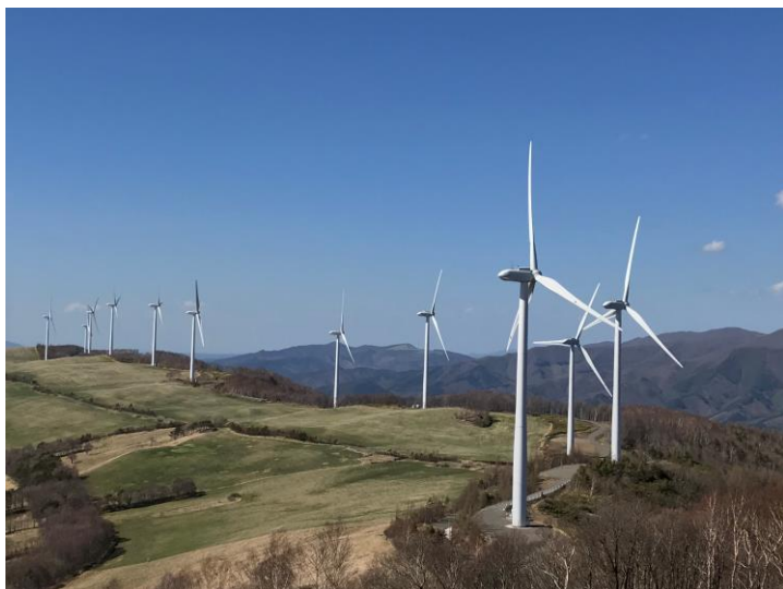
Kuzumaki No.2 Wind Farm (Iwate Pref. 44.6MW 2MW×16 units, 2.1MW×6 units)
