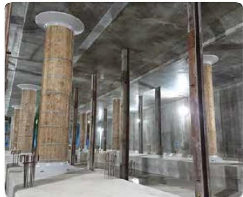
Shin-Yokohama Station (tentative name) on the Through Line between Sotetsu and Tokyu
