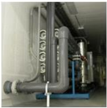
Ion Exchange System
