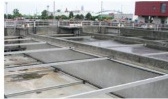
Chain and Fight Sludge Collector
