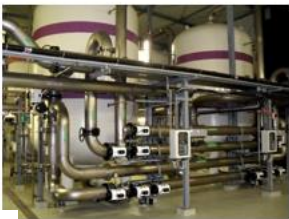
Ion Exchange System
