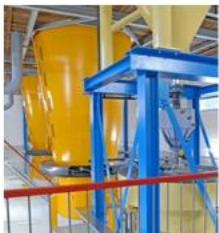
Water Softening System
